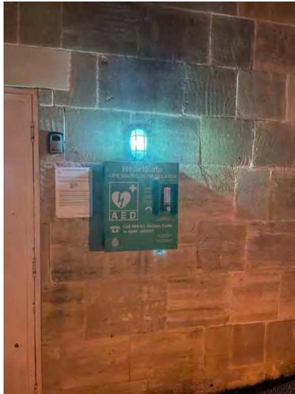
Plate 11. Location/Safety Lighting Highlighting an AED
