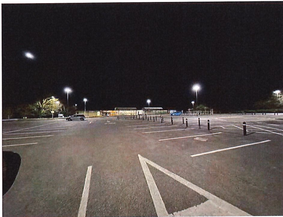
Plate 14. Car Park /Security/Shop Lighting at Sainsbury's Car Park
