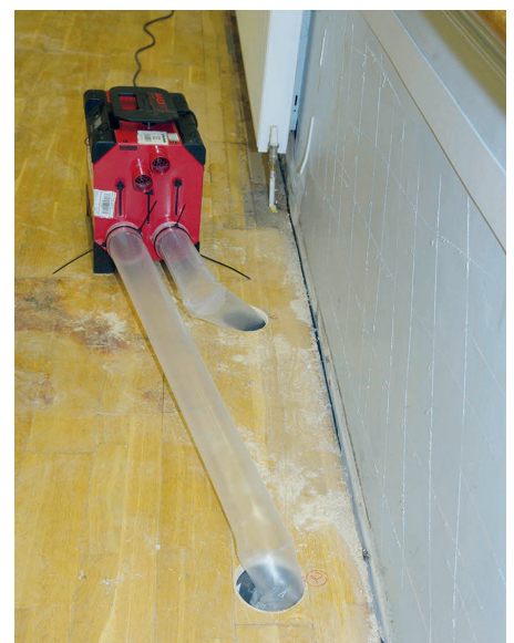
■ Dehumidifiers are in place at St Margaret's Hall, working round the clock to force warm air into the space below the floor
