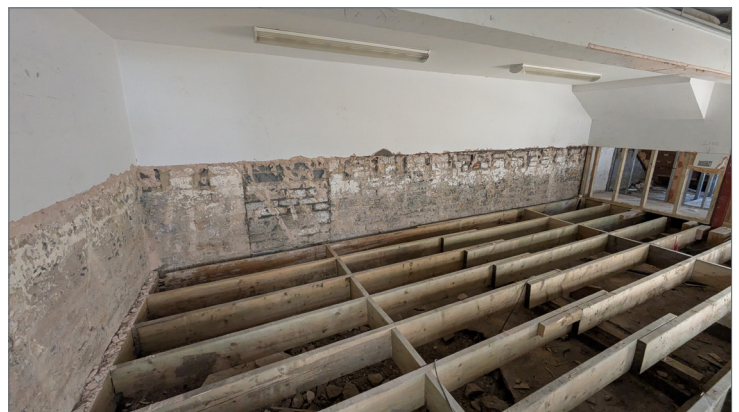
Backstage in St Margaret's Hall with the water-damaged floor removed
